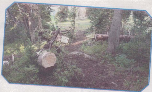
COURTESY PHOTO | COPMOBA.ORG Volunteers with COPMOBA spent a day building and improving the new Mesa Top trail on the Grand Mesa.
